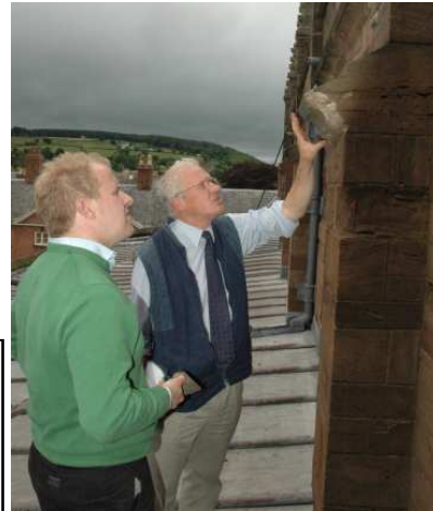
New clerks of works Shaun Ward inspects recently damaged stone-work on the nave of St Laurence's with newly appointed retained builders Stephen Treasure of Treasure's.
